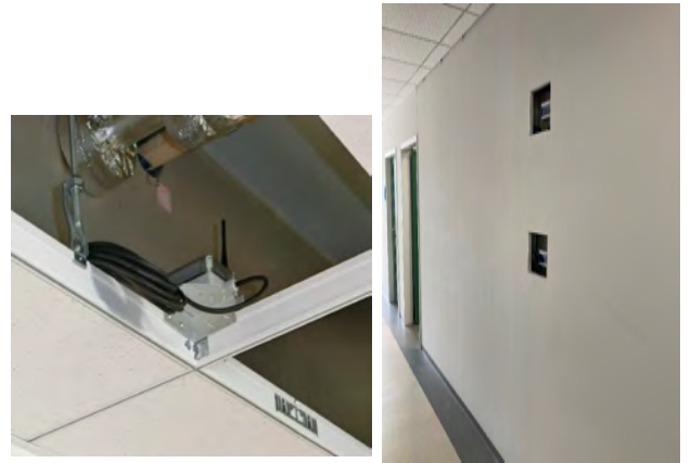
Figure 4-31 Accelerometers on the Ceiling (Left) and Non-structural Walls (Right)
